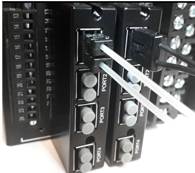
Figure 21: Arc Flash Sensors connected to the 8 Series relay
